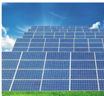
On - Grid Solar Power Plant
