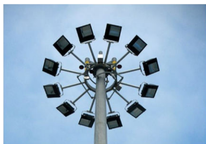
Solar Street Light- High Mast
